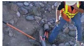
Arizona fiber trunk vandal 2015
